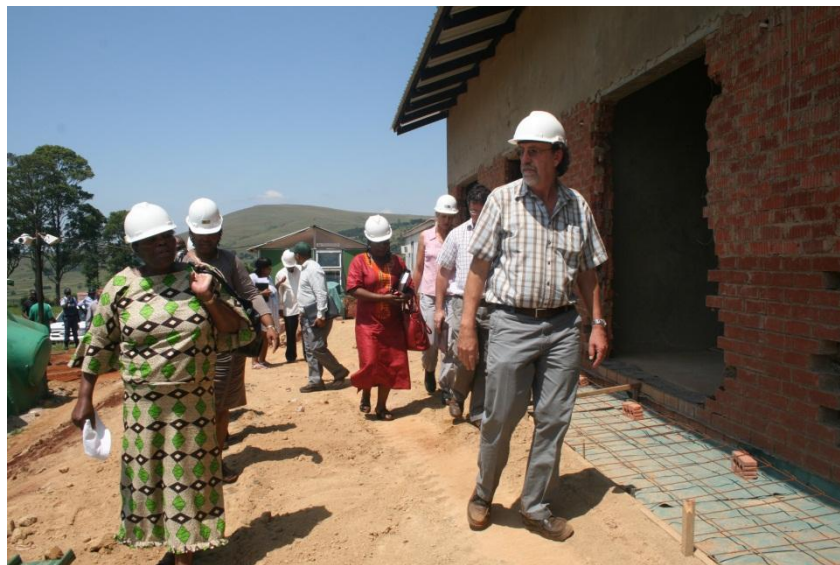
Members of the Portfolio Committee being given a tour of the construction site by the contractor
