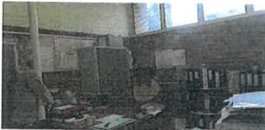
Image 9 Interior condition open plan offices of SCM building (Source: Author)
