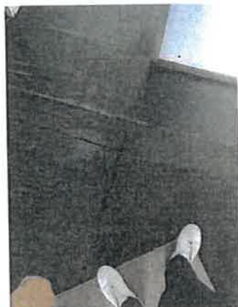
Photo: poor floor: MMC
